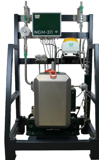
Installed NGM-311 with a pump
